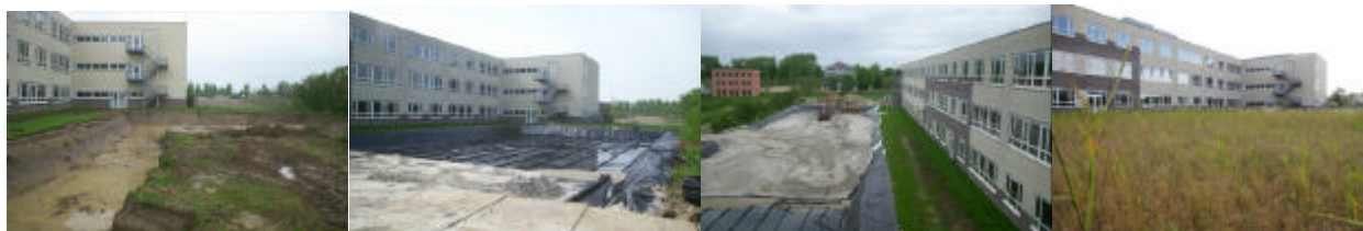
Excavation 1 m deep Foils, shells and lava Clean sand filling Drip pipes and reed
